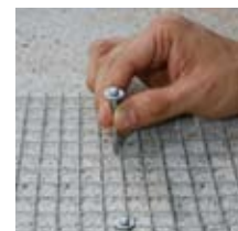
Close up of drive pin anchoring the reinforcing wire after being driven through metal slug and into concrete.
